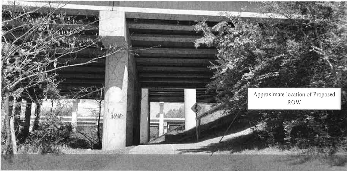
Photograph #1- Bob Callan/Rottenwood Creek Trail- View of existing trail under I-285 where required ROW is proposed and express lanes are to be constructed above the trail. Photographer facing north.
